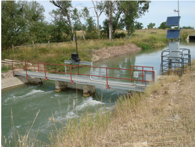
Figure 3-2. Gate Automation Unit Installed in the Belle Fourche Irrigation District.
